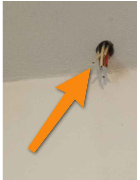
Low Voltage Wires Exposed - Laundry Room
