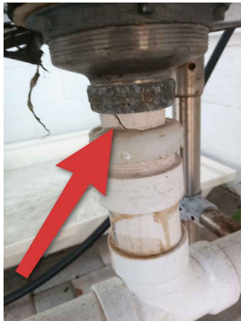
Crack in Pipe - Under Right Sink
