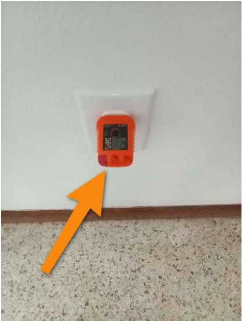
Inoperable Receptacle - Nearest Front Entry Door
